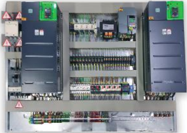
ELEKTRİK PANOLARI / ELECTRICAL PANELS
